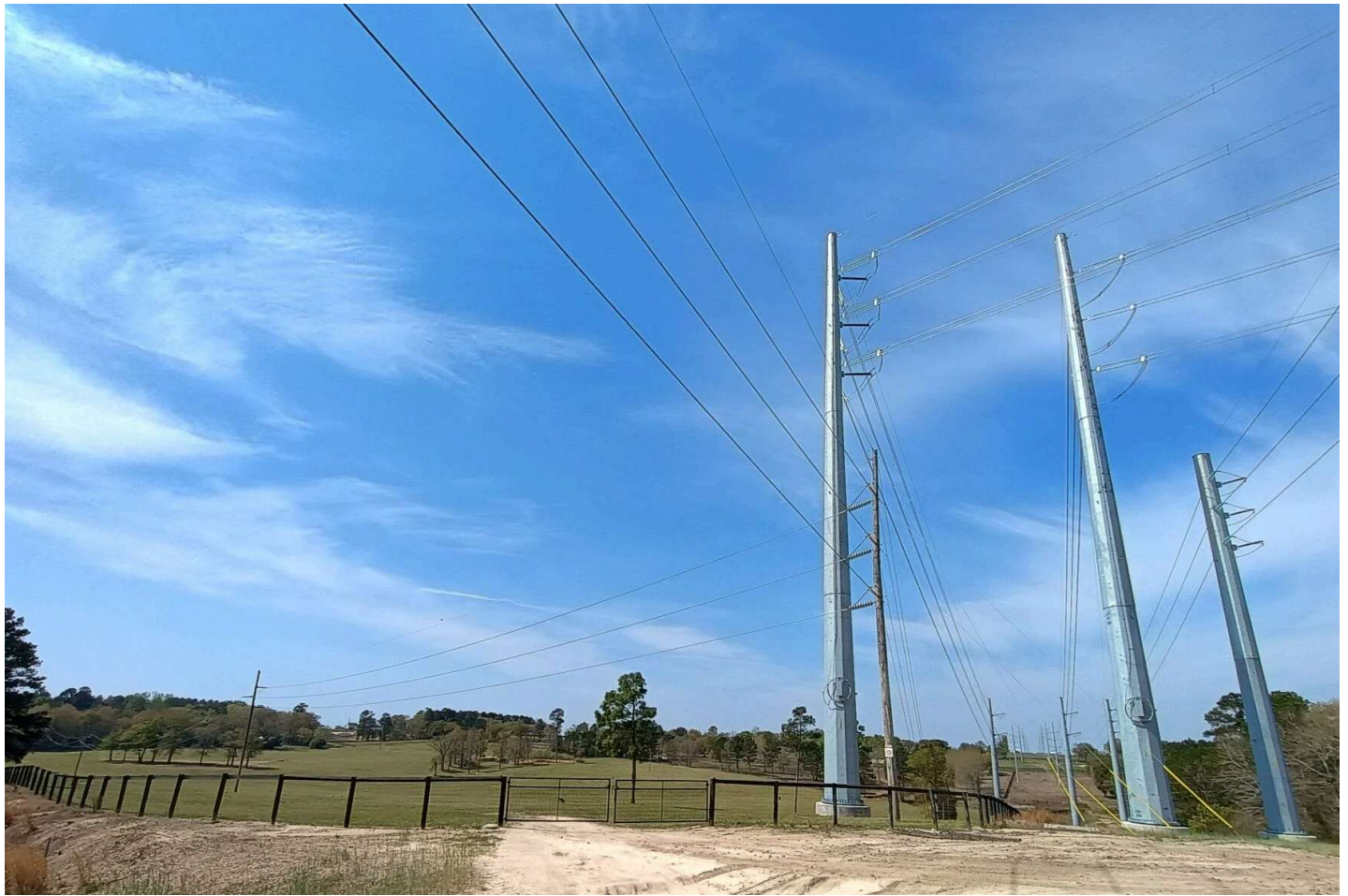
Power lines to a substation off New Holland Road near Aiken, target of land speculators interested in building a new gas plant.
